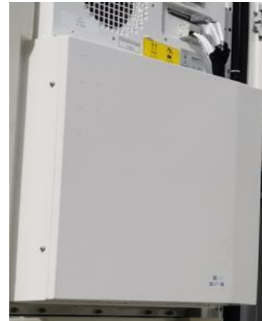
Air conditioner in the ESS
