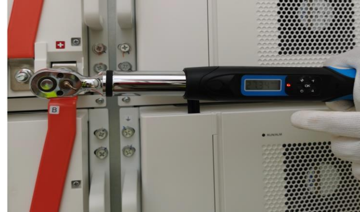
Copper bar connection
